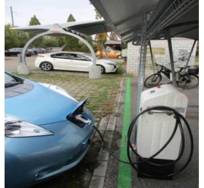
EV charging at PV LAB (CH)
